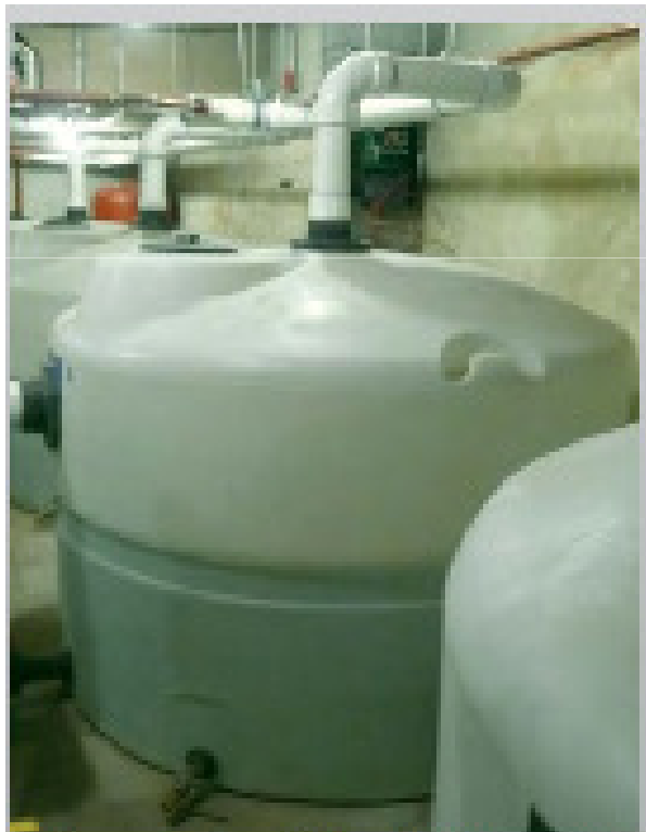
Cisterns operate as part of a rainwater harvesting system in Philadelphia that collects roof runoff for uses such as landscape irrigation or water reuse.
